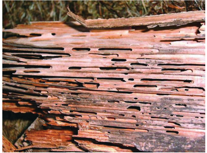
Figure 10. Carpenter ant damage to wood. Credits: www.wdiohio.com
