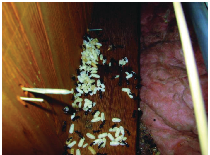
Figure 9. Carpenter ants in an attic space. Credits: portlandhomeinspections.com
